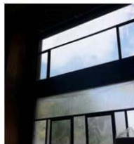
BEL Replace fogged window panes
